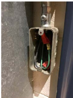
Exposed Junction Box (Stage)
