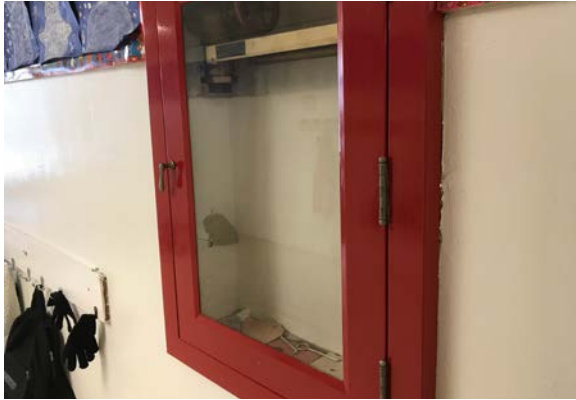
Fire Hose Cabinet
