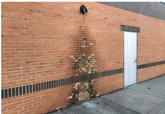
Brick (water damage)
