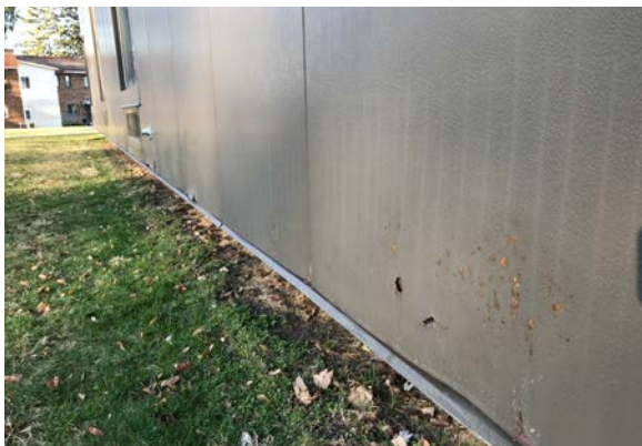
Metal Panel Corrosion
